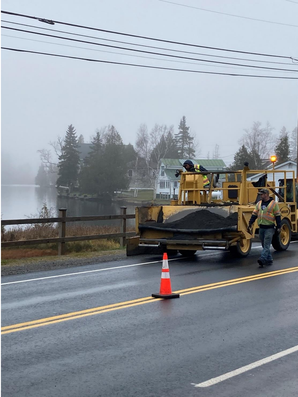
Photo of crews placing aggregate shoulders at Joe's Pond in West Danville.
