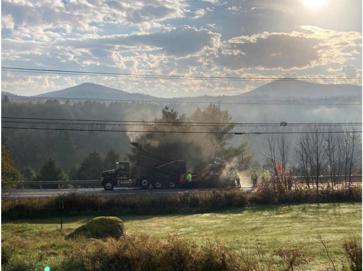
Photo of crews paving a section of roadway near Eaton Cemetery Road that was damaged by a truck accident.
