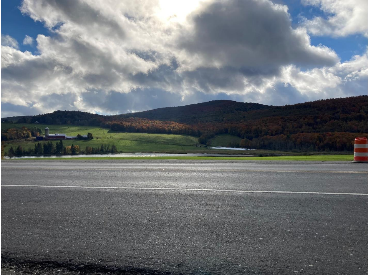
Photo of a section of roadway awaiting to be paved on U.S. 2 in Cabot.
