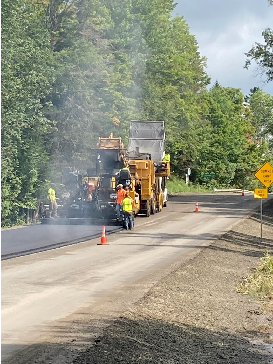
Photo of crews paving the last gravel section near Joe's Pond in West Danville.
