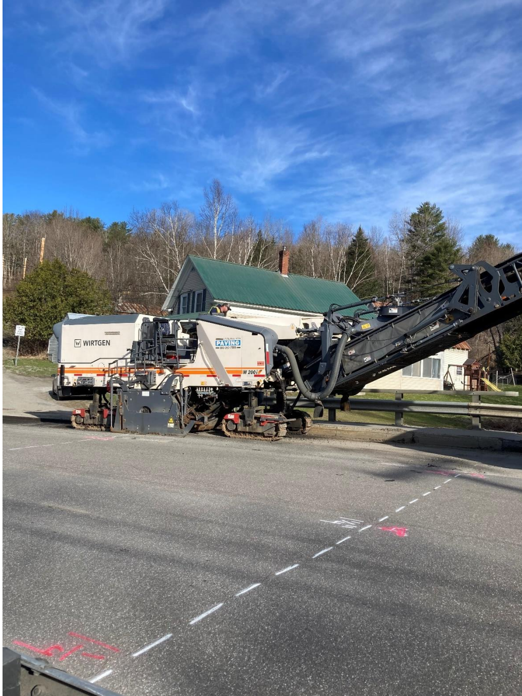
Photo of the milling of pavement on Bridge #80 on U.S. 2 at the intersection with English Cemetery Road
