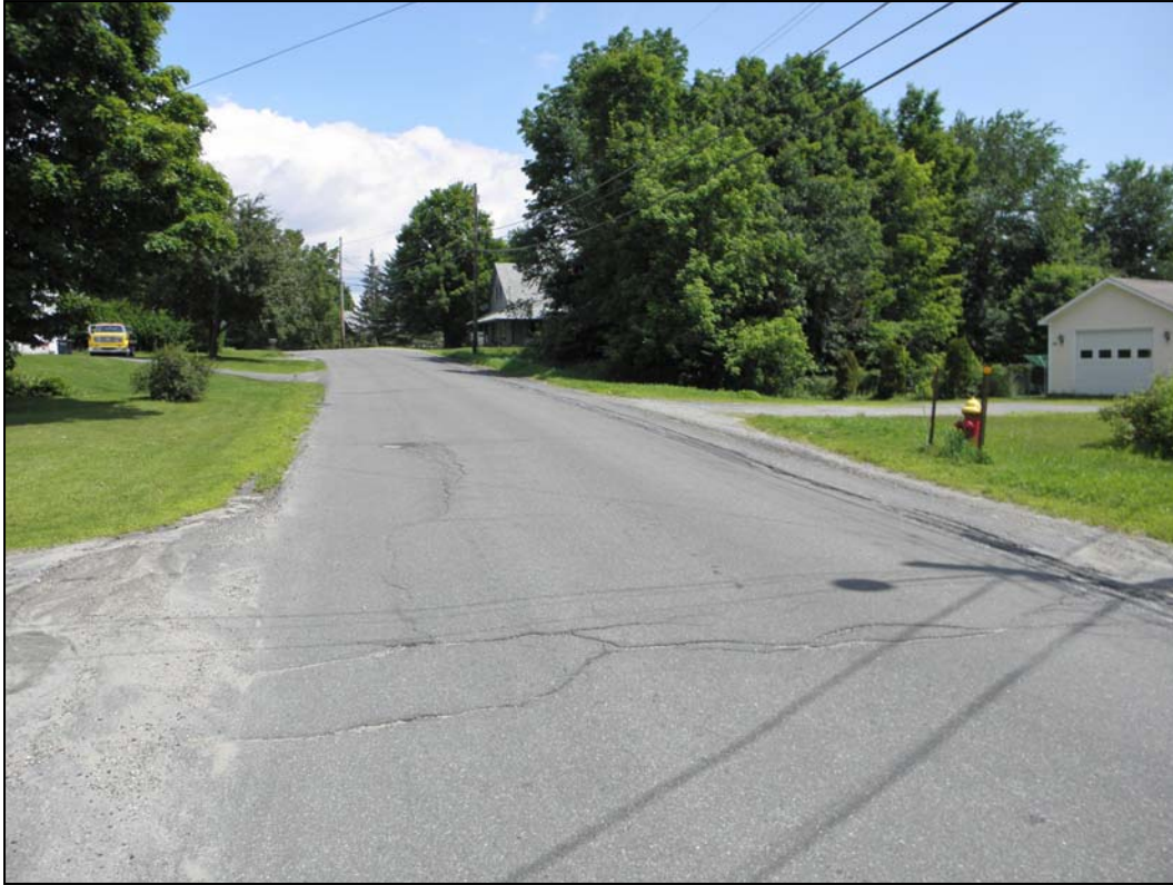
Photo 20. Peacham Road with hydrant on the right and storm drainage swale on the left. View to the north.
