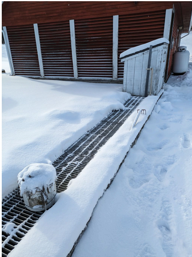
Figure 2-7: Headworks Channel & Influent Sampler
