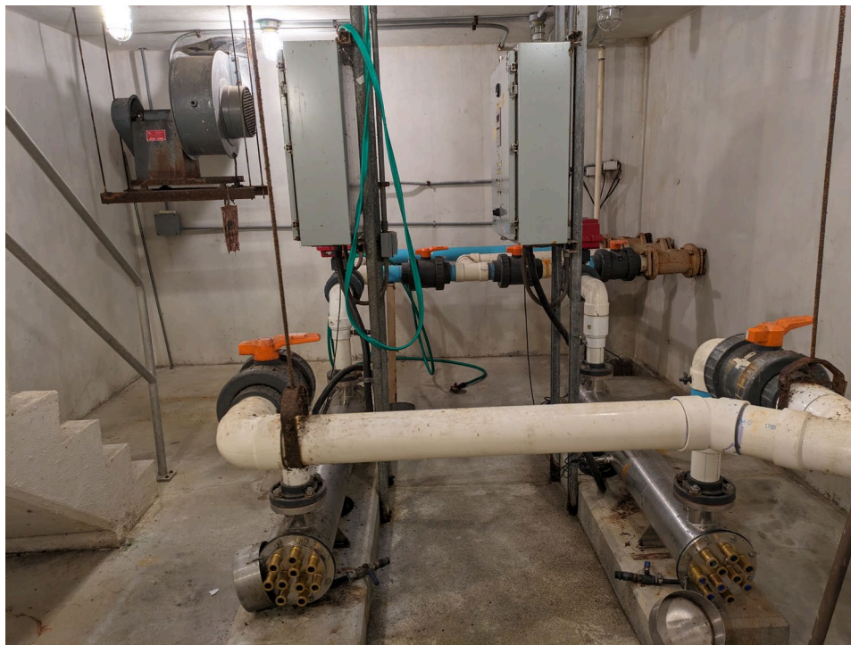
Figure 2-10: UV Disinfection Systems & Control Panels
