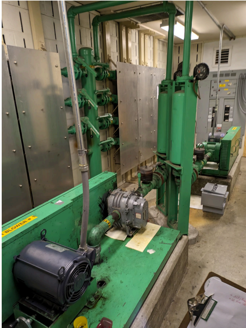
Figure 2-9: Aeration Blowers & Discharge Manifold
