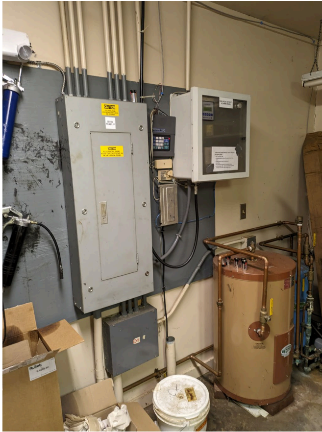
Figure 2-12: Electrical Service & Water Heater
