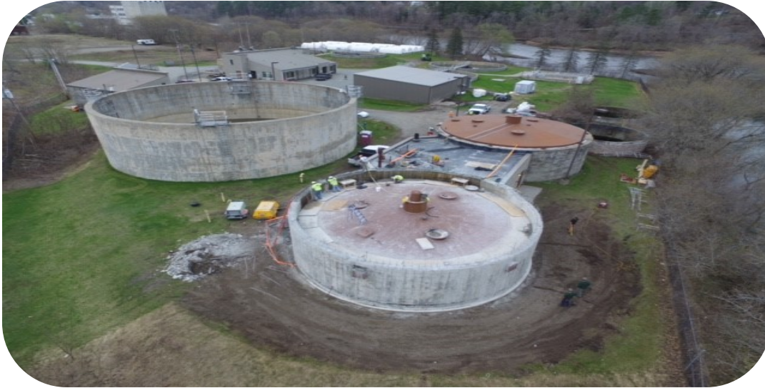
St. Johnsbury Wastewater Treatment Plant
