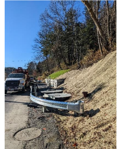
New Submersible Station
